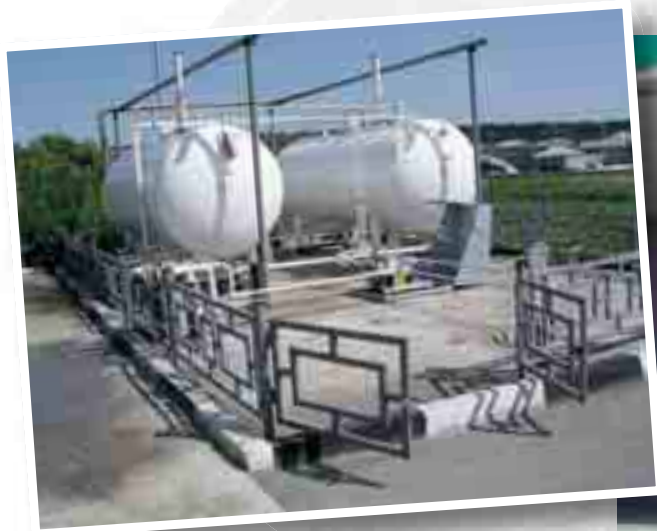
Aboveground autogas installation using one autogas series pump with two tanks.
