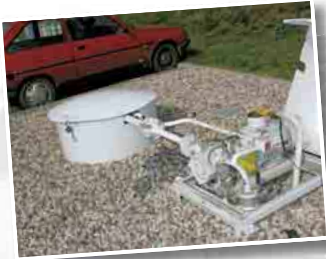
Underground autogas installation using one autogas series pump with one tank.
