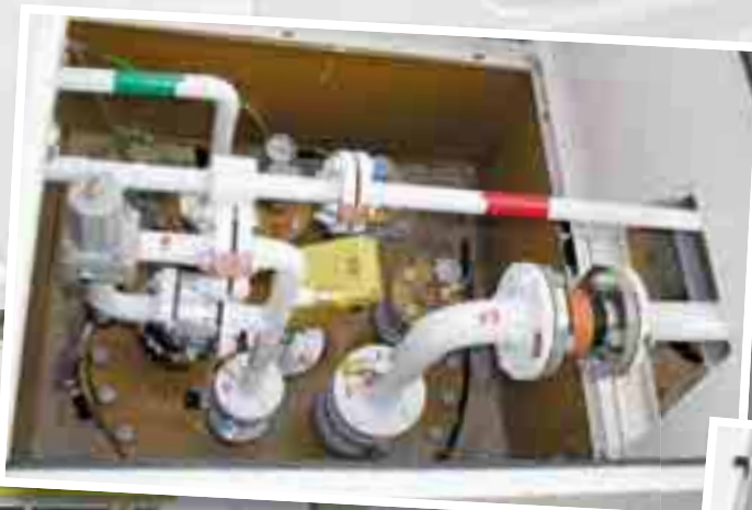
Underground autogas installation using one autogas series pump with one tank.
