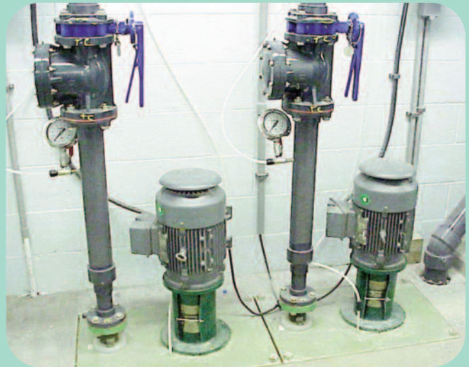
Fybroc Series 5500 Vertical pump installation
